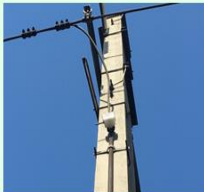
Suction line monitoring
